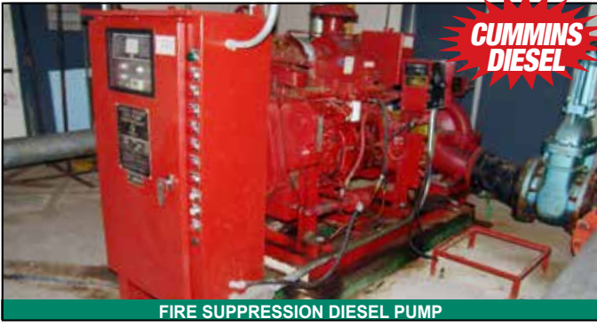
FIRE SUPPRESSION DIESEL PUMP
