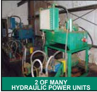
2 OF MANY HYDRAULIC POWER UNITS
