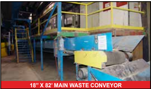
18" X 82' MAIN WASTE CONVEYOR
